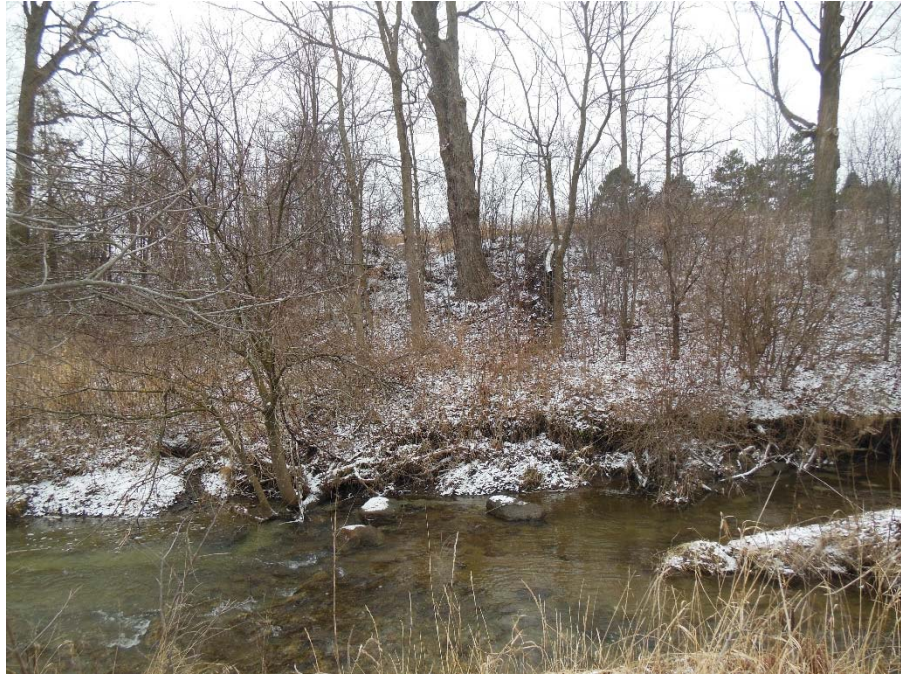
Undercutting at toe of slope adjacent to Borehole 16-2
