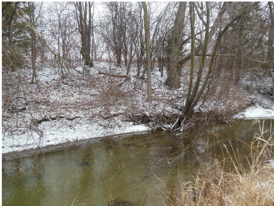
Undercutting at toe of slope leads to bank erosion adjacent to Borehole 16-2
