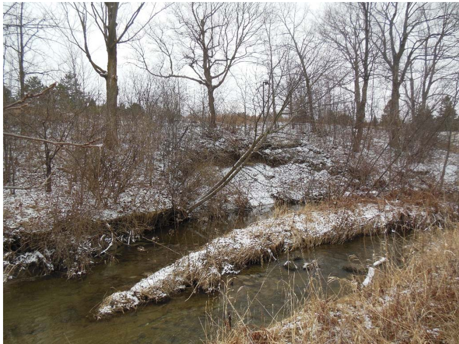
Local sloughing of slope adjacent to Borehole 16-1 looking to the north
